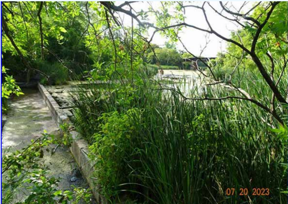
Downstream face of the Lake Washington Dam. Note the floating cattail bogs at both the right and left abutments.
