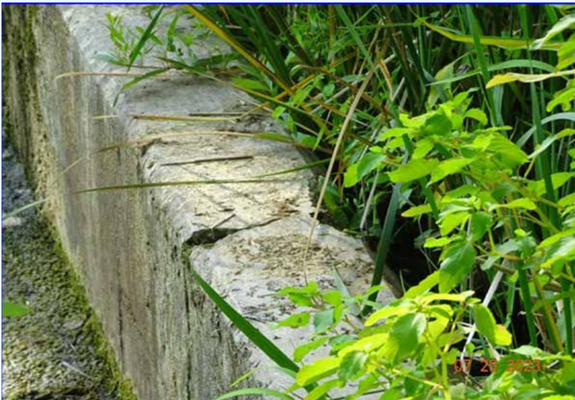
Crack in the concrete approximately five feet from the left abutment. Note the scour and vegetation on the upstream side of the weir.
