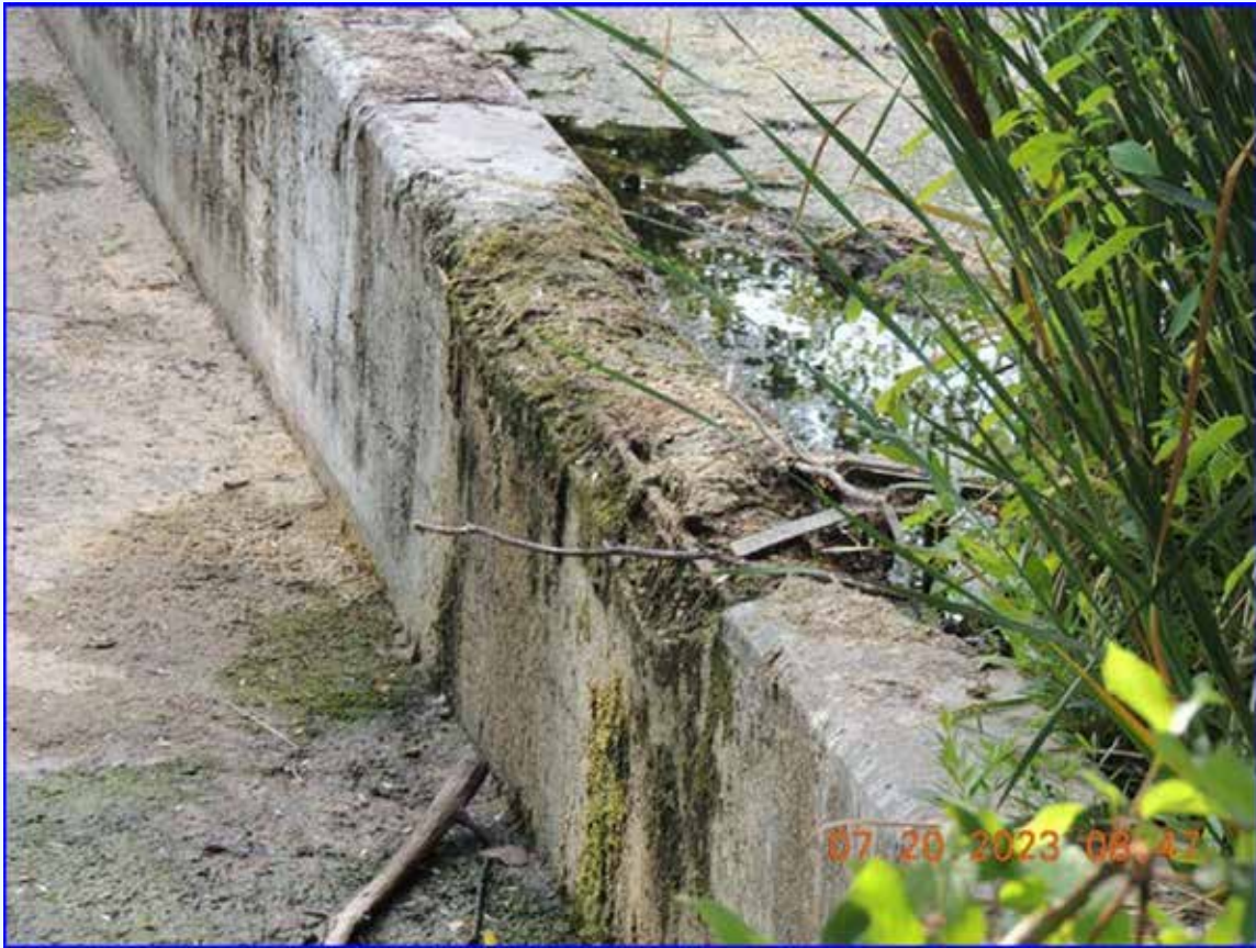
Concrete scour near the left abutment. Note the exposed rebar. Remnants of the steel carp barrier post can be seen on the lower right of the scour.
